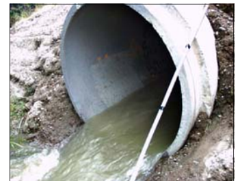
Storm water outlet releasing sewage.
